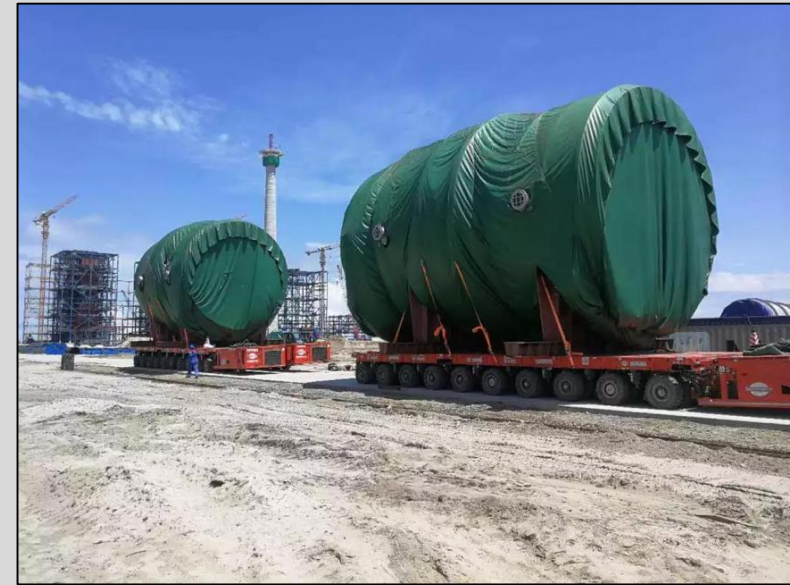
Hengyi Petrochemical & Refinery Plant
