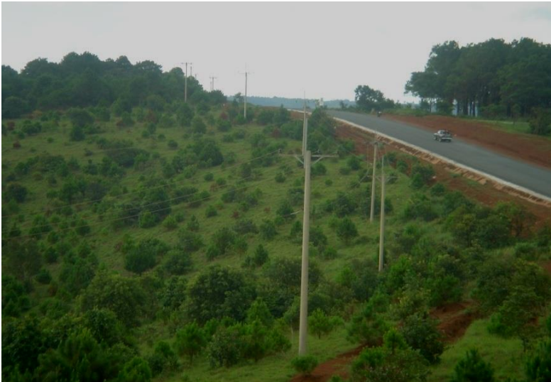
22 kV MV Line at Mondulkiri Province
