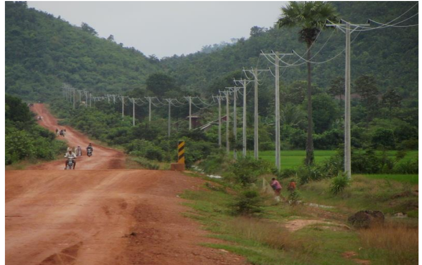
22 kV MV Line at Kampot Province
