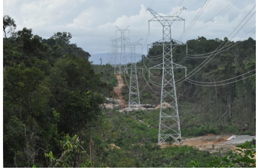
Posat – O Soam 230 kV Transmission Line
