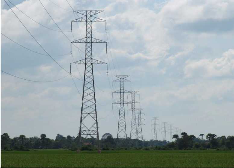
Takeo – Kampot 230 kV Transmission Line
